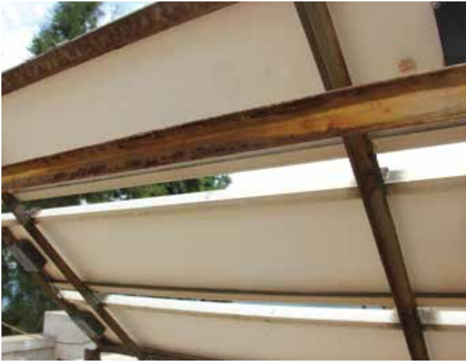
The frame and rack are rusty, but the DuPont™ Tedlar® PVF film-based backsheets are in excellent condition after 20 years of outdoor exposure. The PVF film on the back of the modules shows minimal yellowing, illustrating the excellent weatherability of the film
